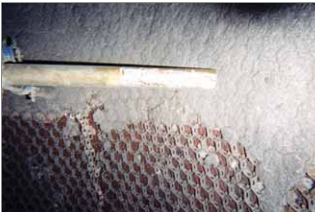
Figure 1. Material worn through.
